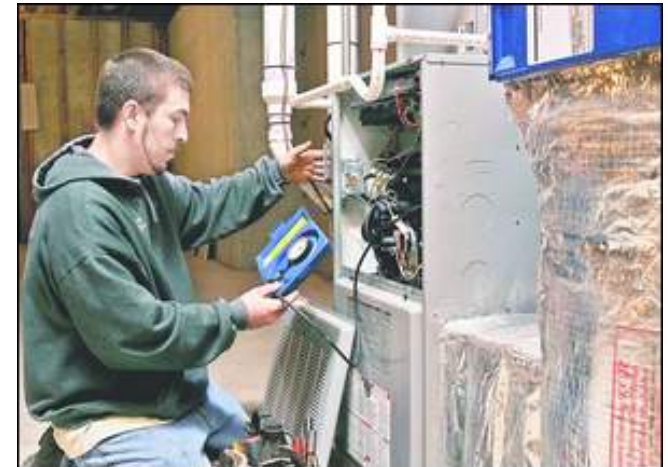
Denise DeVore/For the Journal Before winter arrives, make sure your furnace is working properly. Check that the air filter is clean and all hoses are tight. Arthur Davies of Airflow Air Conditioning in Milton checks a furnace for problems.
